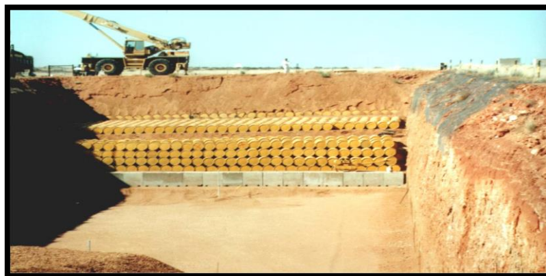
Figure 4 : The Sealed Containers are Packed into Near Surface Bunkers for Long Term Storage
