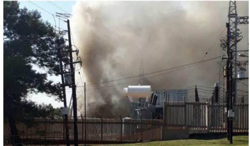
The Mooikloof substation goes up in flames.
